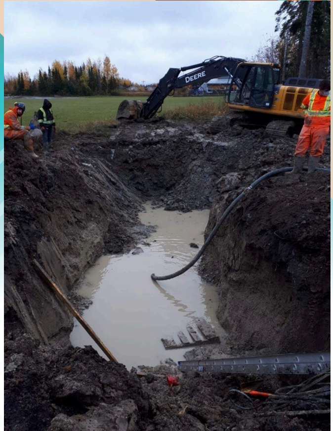
Photo courtesy of Red Lake Plumbing and Heating
